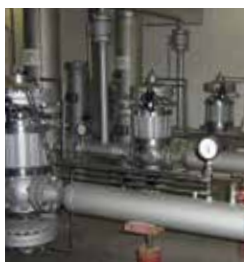
CABINE DI PRIMO SALTO HIGH PRESSURE REDUCING & METERING STATIONS
