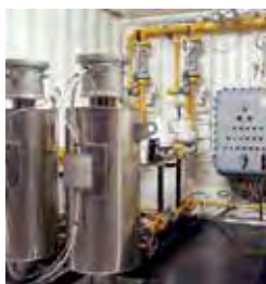
STAZIONI CNG VIRTUAL PIPELINE CNG DAUGHTER STATIONS VIRTUAL PIPELINE
