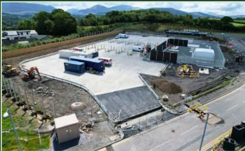
6 months since ground works commenced, we're now well underway with our first concrete being poured — 70%
