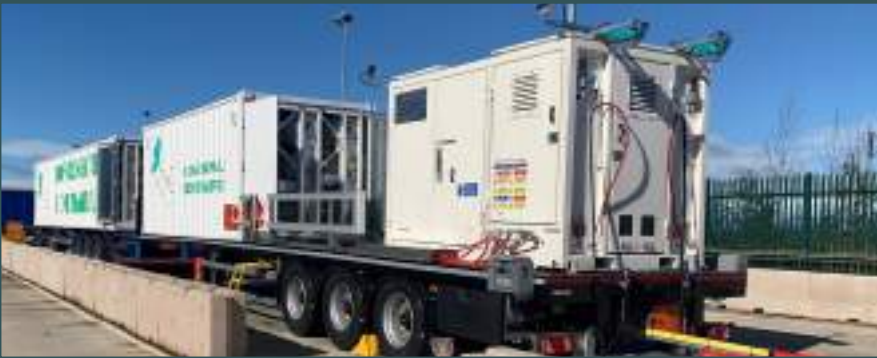
MRU set-up at a customer site
