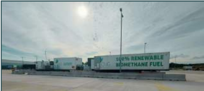
A closer look at the easy mobile re-fuelling depot based at a customers site
