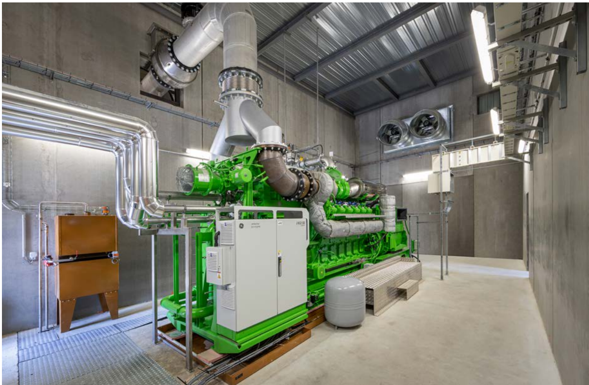
Picture: CHP unit for power and heat generation
