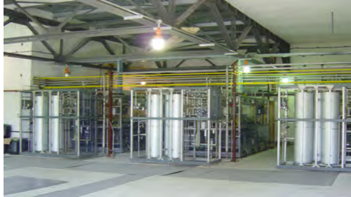
Hydrogenics electrolysis plant in Ukraine
